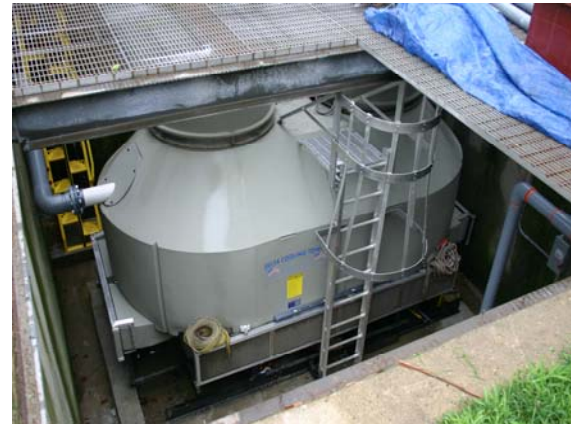
The 250-ton Premier tower chosen to cool the museum area of Lady Liberty
