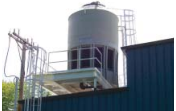
Cooling water flows through an open loop while process water flows through a closed loop to the cooling coils in the induction heater, and back again.
